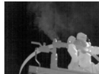
Captured SF 6 leak
