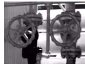
Capture gas leak from production site
